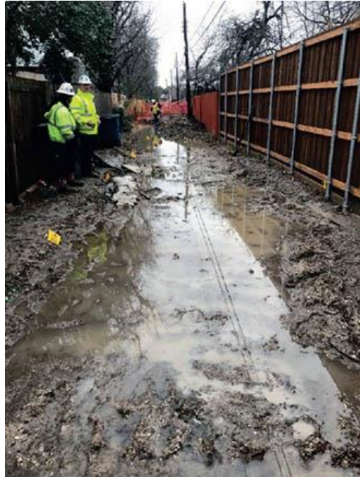
Figure 7: Water Saturated Ground with Puddling
