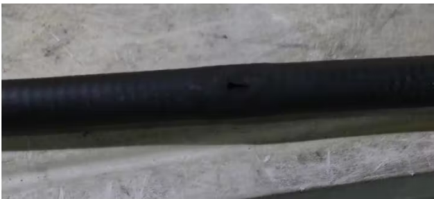
Figure 6 Post Test Visual Assessment – Arc Resistant Jacket CSST
