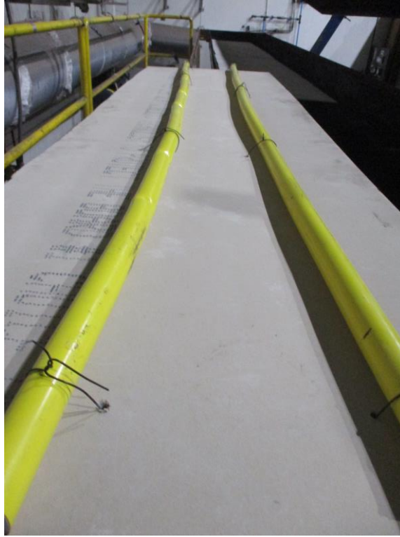
PEXALGAS Metal Tubing 32 x 3 Pre-Test
